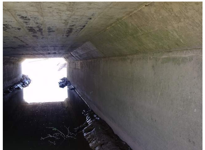
West Surface. Showing isolated cracking.
