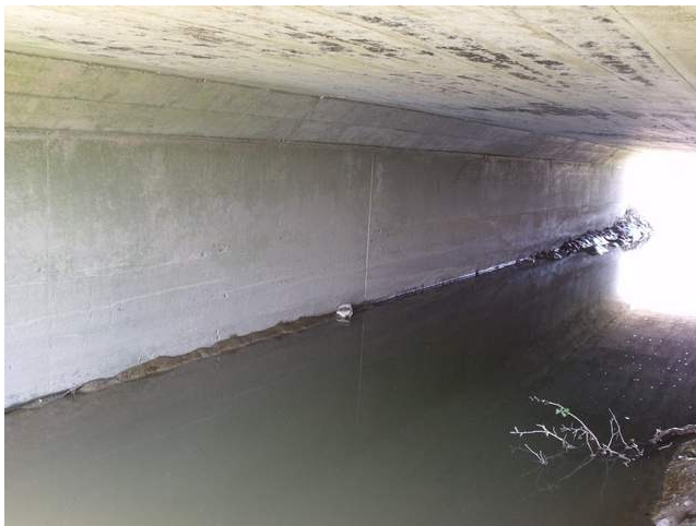
East Surface. Showing isolated cracking.
